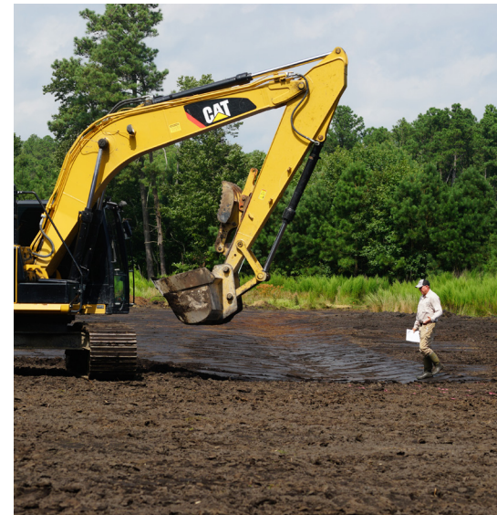
DWL's Ron Haas on site during construction of one of the Long Field swales.
