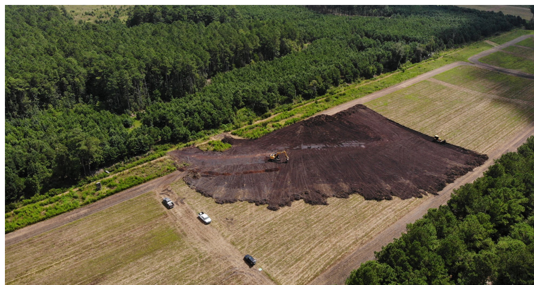
Earthwork is underway for our 80-acre Long Field restoration. Note our Field 7 wetland restoration site visible in the upper left portion of the photo.
